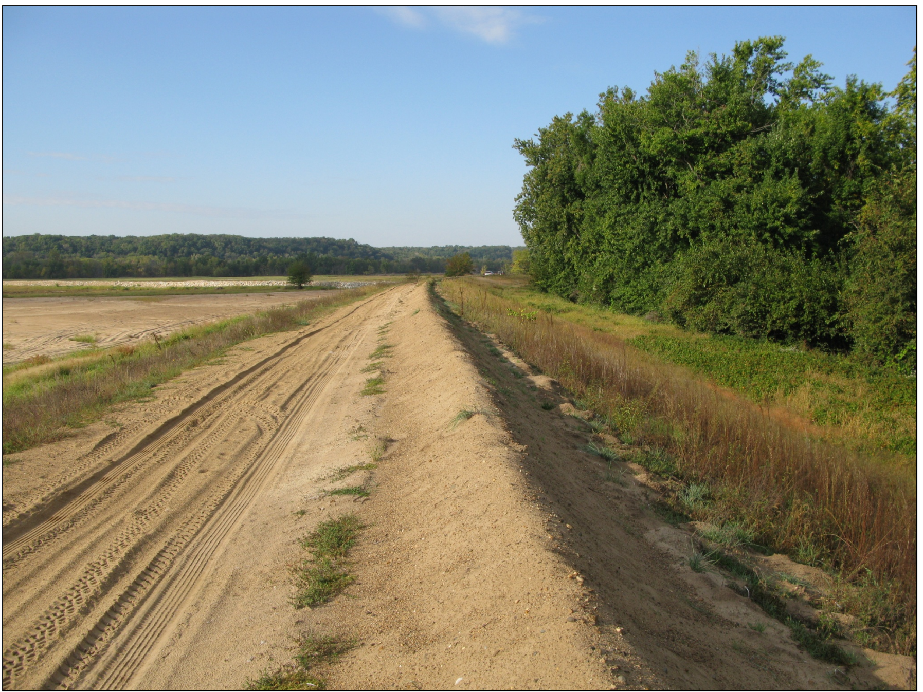
Example “push-up” (plastic sheeting has disintegrated in the sunlight)
