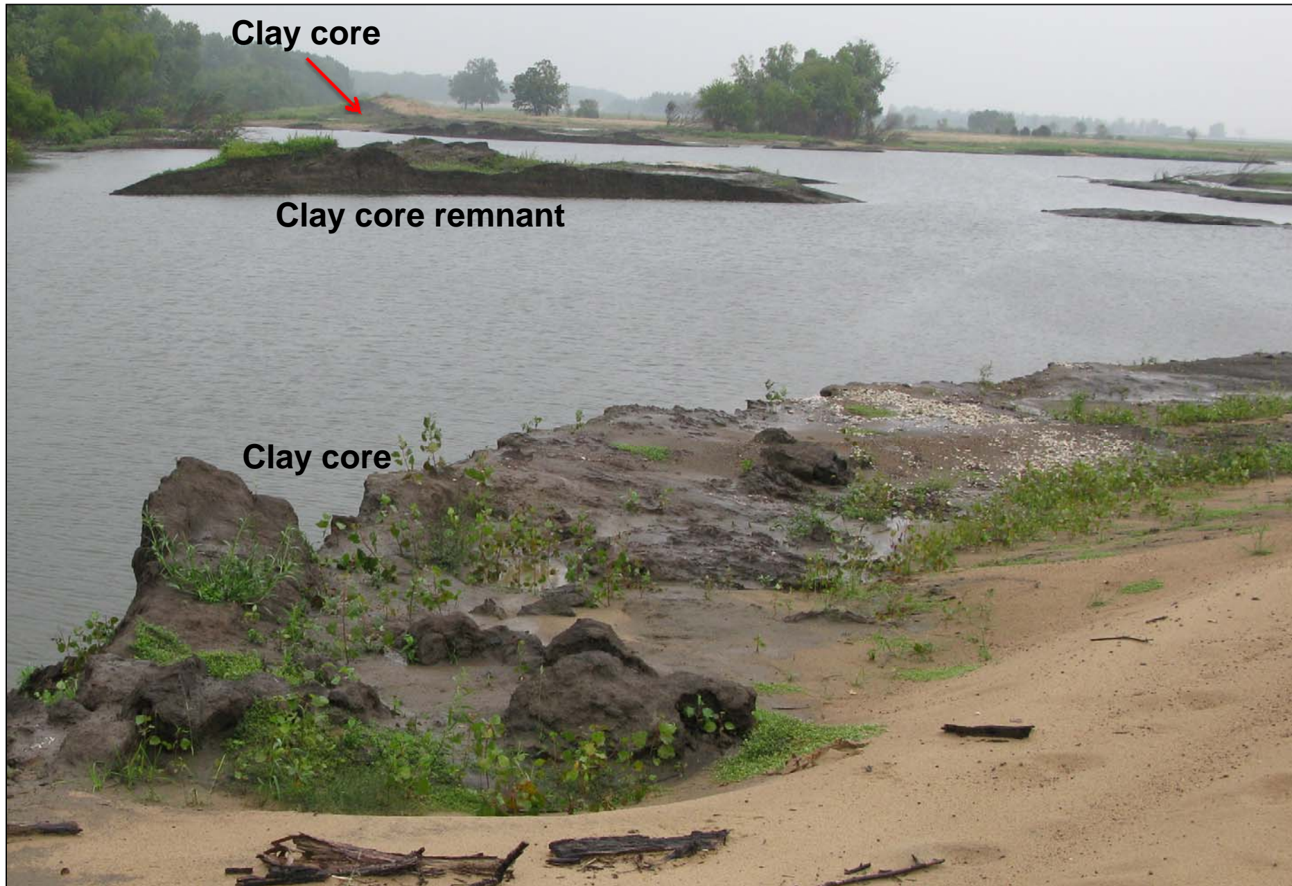
Main 2008 break was over 1000 ft. wide and the resulting scour hole ~35 ft. deep
